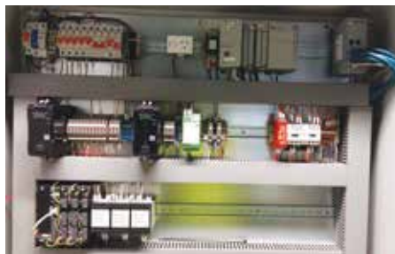
• PLC panel inside
