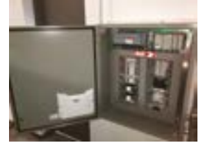
Georgia Pacific – Dudley, NC, USA Commissioned: March 2018
