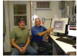
Jeff (left) and Ray (Right) Wheeland seen here with the new A&E control system.
