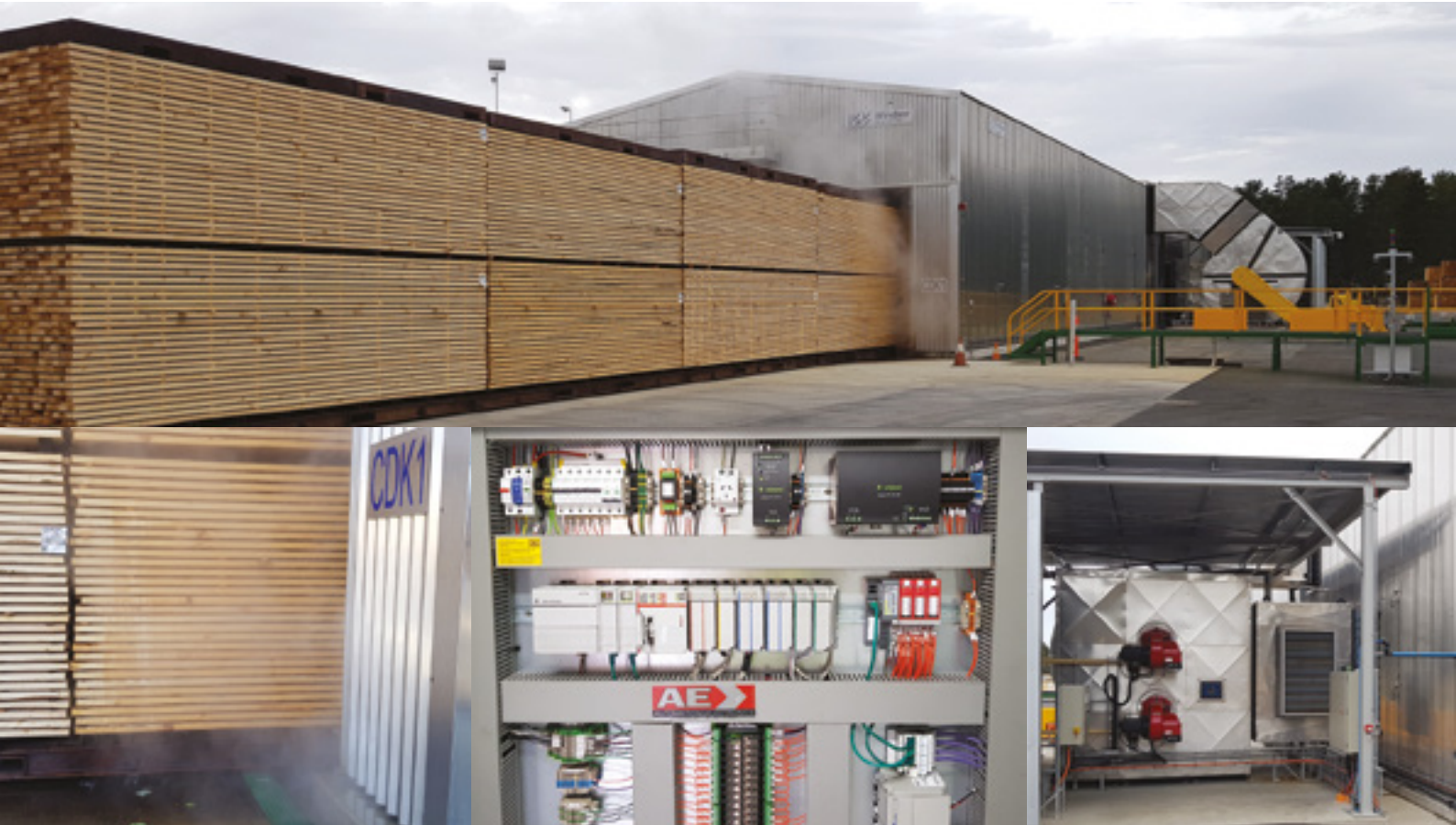
Pictured: TOP: Wide view of the Westpine CDK Kiln in action BOTTOM: Right & Left are all close up shots of the Kiln in action. Central pic is a close up shot of the controls installed by A&E.
